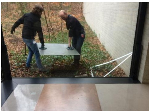
Head of technical department Frank Meijerink and Bjorn Tuinstra during the installation of Copper inside-outside piece at the Kröller-Müller Museum in 2018. Photo: © Jip Hinten
